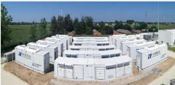
40MW/40MWh Huaneng Wind Energy Storage Frequency Modulation Project
