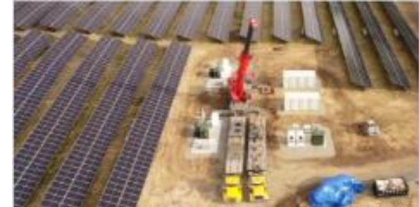
21.6MWh Energy Storage Project in Massachusetts, USA
