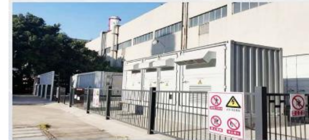
Shenzhen Nanshan Power Plant Frequency Modulation Project
