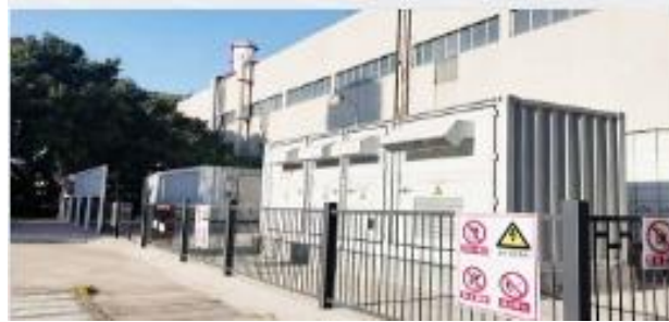
Shenzhen Nanshan Power Plant Frequency Modulation Project
