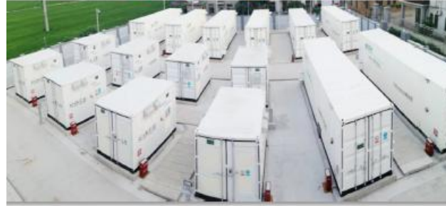
8MW/16MWh State Grid Zhenjiang Changwang Energy Storage Project
