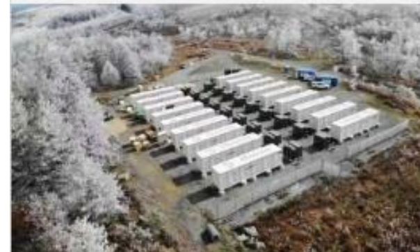
72MW/72MWh PJM FM Project in the United States
