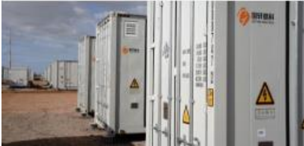
492MWh Energy Storage Project in Arizona, USA
