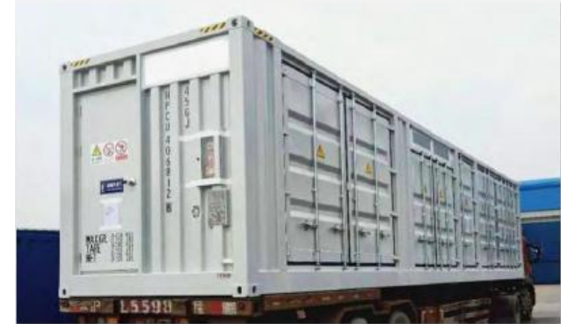
Dubai Light Diesel Storage Microgrid Project
